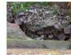
L. DRAINAGE BEHIND WALL - HEAVILY IMPACTED
