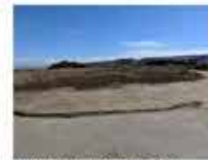
J. MOUNDED PLANTING AREA - EROSION CAUSING SILT/DEBRIS
