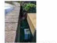
H. WATER NOT GETTING BEHIND WALL WITH DRAINAGE STRUCTURE
