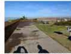
D. WALKWAY TO OUTLOOK AREA - DRAINAGE NOT WORKING
