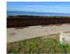
C. WALL DRAINAGE STRUCTURE - MINOR PONDING
