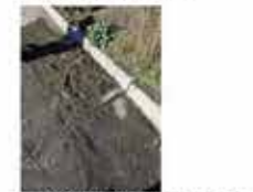
N. PARKING LOT DRAIN - CLOGGED DURING FIRST RAIN EVENT
