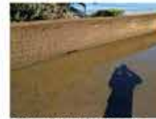
G. DRAINAGE STRUCTURE - NOT WORKING CORRECTLY
