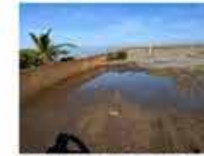
F. DRAINAGE STRUCTURE - NOT WORKING CORRECTLY
